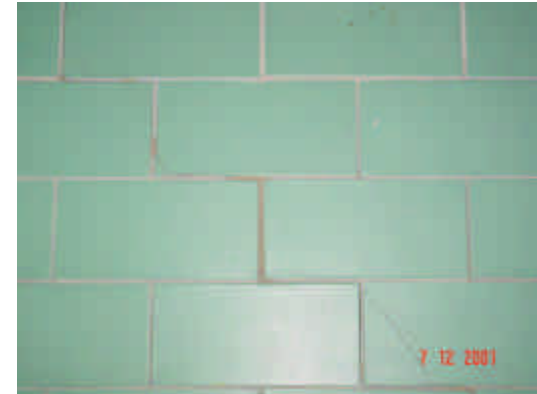
N17-P_SP2 Crack on the north-east corner block wall of pool.
