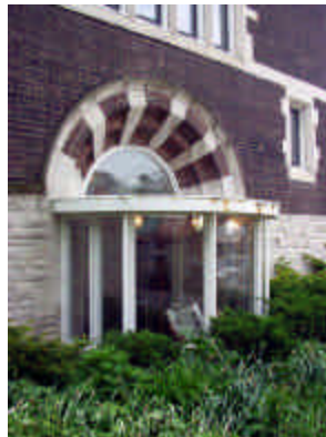
S02_AP11 Rust on metal fascia of the semi-circular reading alcove on north side.
