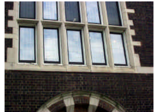
S02_AP09 Restore/replace deteriorated stone window sills. Paint and caulk.
