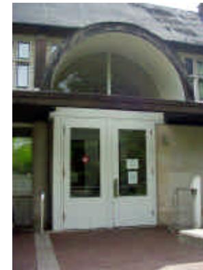
S02_AP12 Front door should be replaced. Paint fascia.
