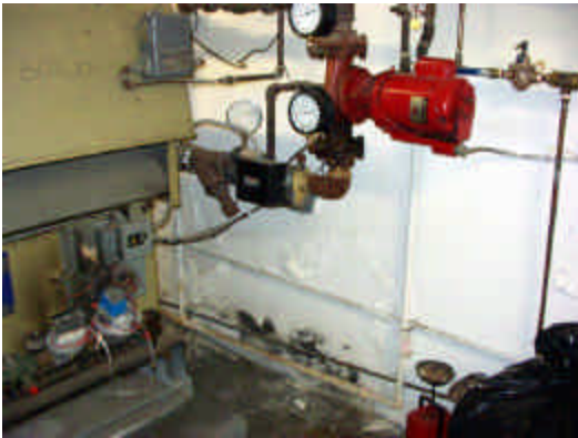
S02_AP15 Water migration to the east foundation wall inside the Mech. Room. The walls have to be painted every 6 months. Excavate and repair weeping tile.
