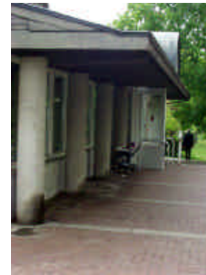
S02_AP06 The paving underneath the canopy is constantly wet,
