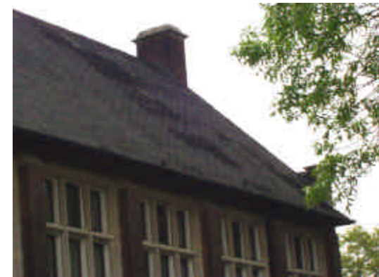
S02_AP03 Roof shingles damaged by pigeons
