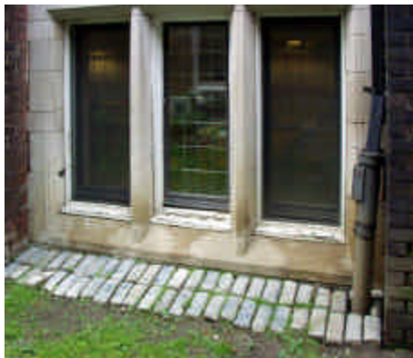
S02_AP08 Restore/replace deteriorated stone window sills. Paint and caulk.
