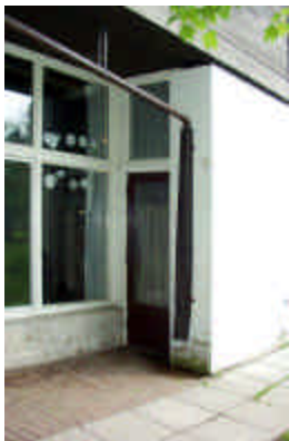
S02_AP07 The south door, window and downspout are constantly vandalised.
